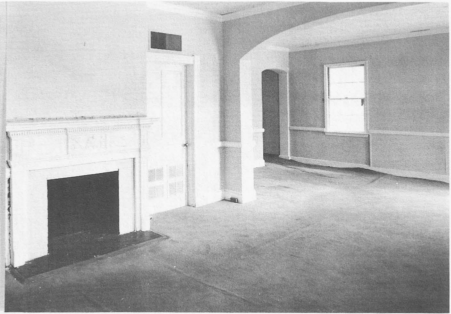
Interior view of reception area in the Moncure Building. The few architectural details in the buildings included this carved wood mantel and gentle ceiling arch, both in the front room.
